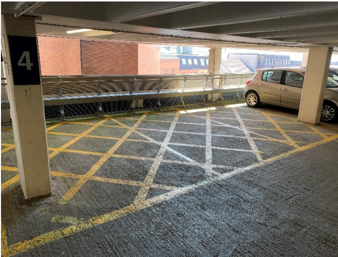
Figure 4 Hatched markings on disabled spaces in Chester Street Car Park making it unclear as to whether they can be used.
